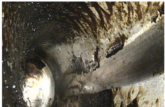
Figure 4 – Hydrocarbon Deposit in Gas Manifold
