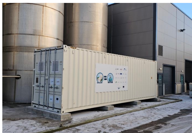
Figure 9: The installation of the AD-BES unit at the demonstration site of Eigerøy, Norway in December 2023
