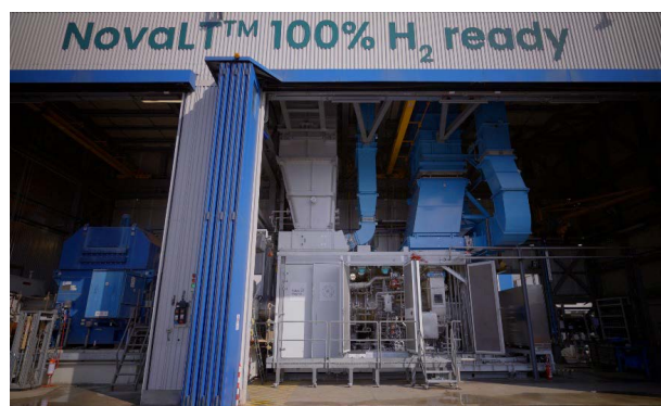
Figure 17 – NovaLT™16 100% hydrogen-ready gas turbine, installed on the Baker Hughes test bench at its Florence site (IT). Image courtesy of Baker Hughes.*
