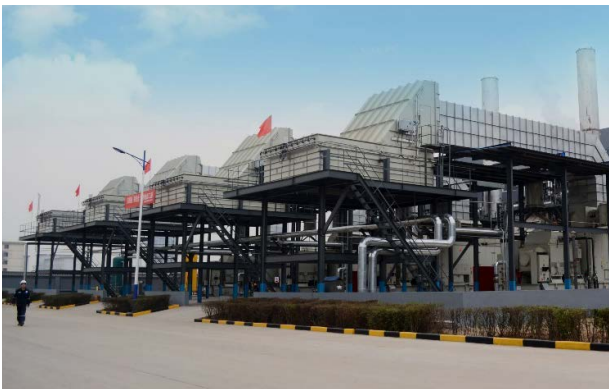
Figure 15 – Titan 130 conventional combustion gas turbine packages operating with up to 65% hydrogen [33].
