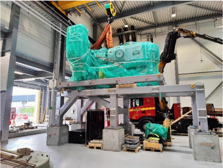
MAN Compressor @ site in Esbjerg
