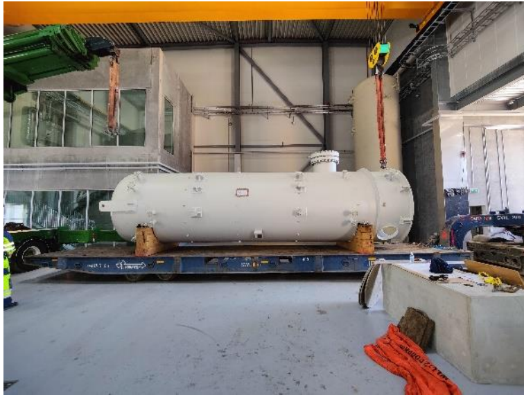
CO 2 storage tank
