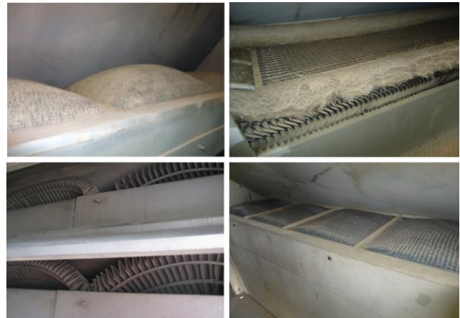
Figure 9, Different types of coalescer filter installed in the weather hoods
