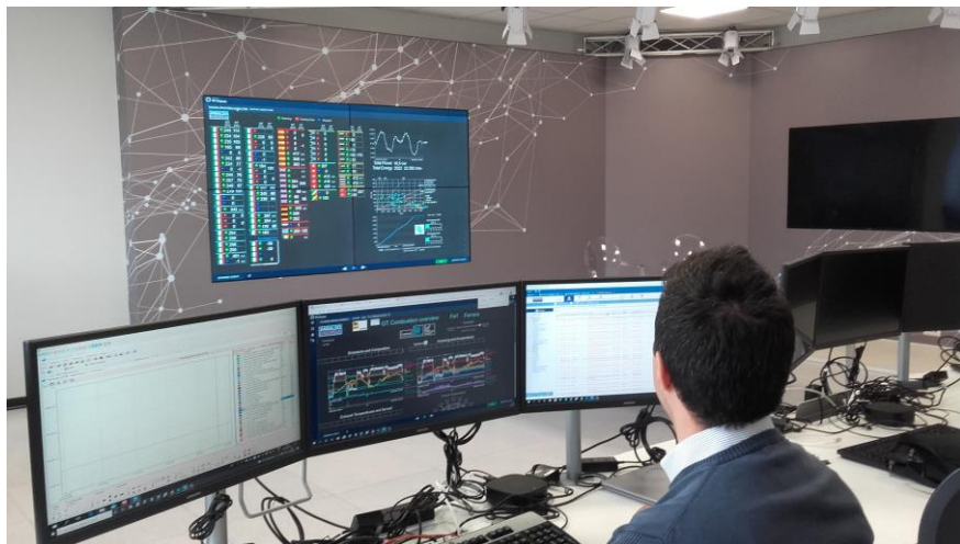
IPS control room in Genoa main AE facility.
