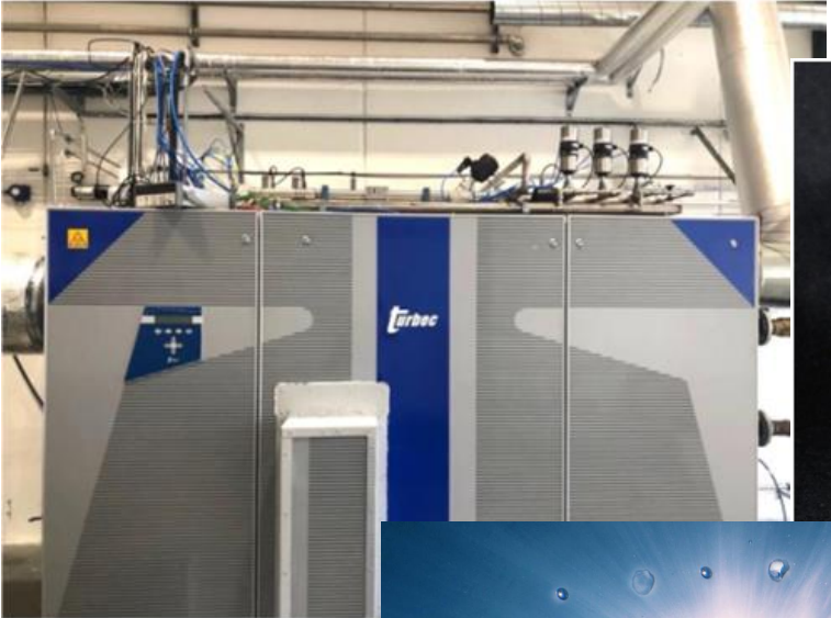
Micro Gas Turbine
