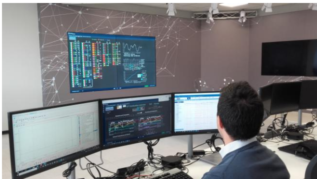
Fig. 5 - IPS control room in Genoa (I) main AE facility.
