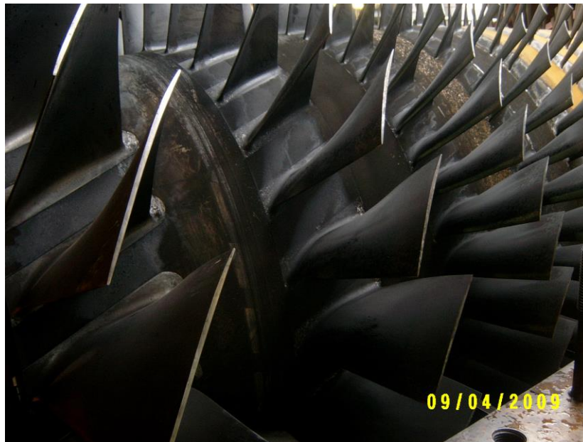
Figure 1: The black deposits on the compressor blades is fouling caused by hydrocarbon contaminants in the atmosphere
