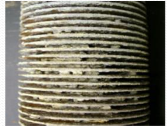
HRSG deposition due to acid dew point (Uniper Technologies)
