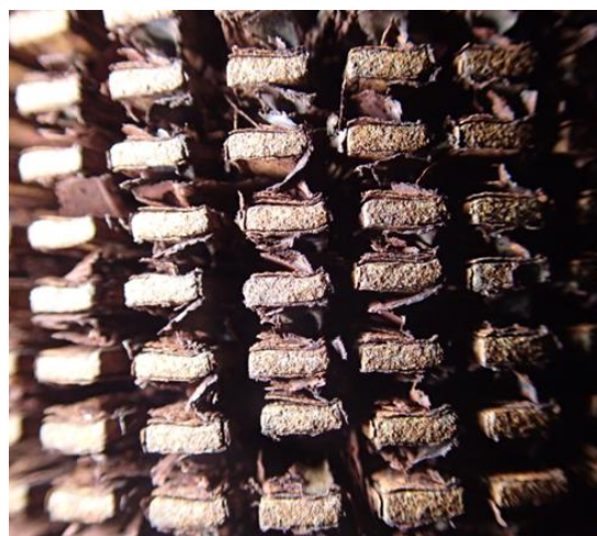
Figure 7: Flue gas side corrosion of finned tube.
