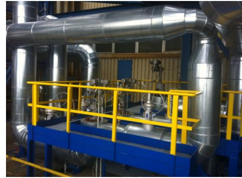
Figure 12: New warm-up HRH steam heating lines
