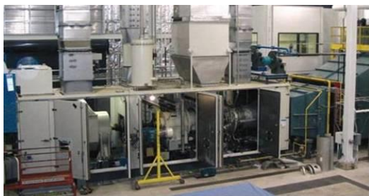
Figure 11: 7.7MW tri-fuel gas turbine installed in a cogeneration plant in the USA
