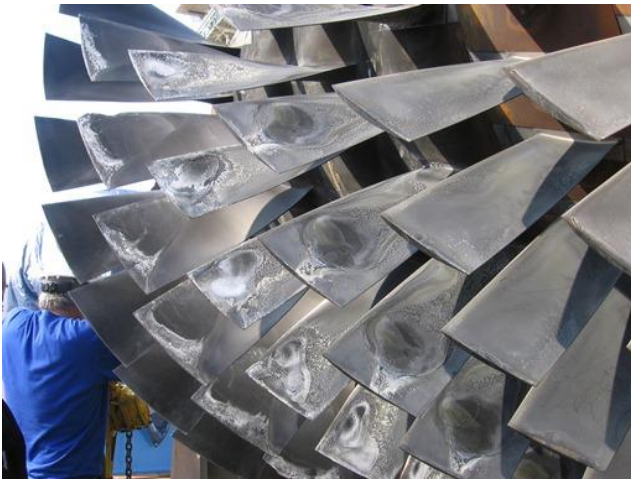
Figure 5. Fouled compressor rotor – black soot, white salt sediments on the first 6 compressor rows.
