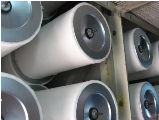
Figure 8. Main filters with wrapped-on pre-filter hoods
