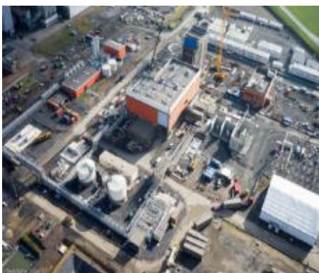
Figure 15. EDF Bouchain Power Plant
