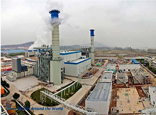
Huaneng Nanjing CC, Configuration 2 X 200-MW, 1+1 CCGT blocks with 9001E gas turbines
