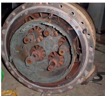
Figure 9: Damages due to high-frequency (2350 Hz) thermoacoustic instabilities due to inappropriate tuning of the machine 23 .
