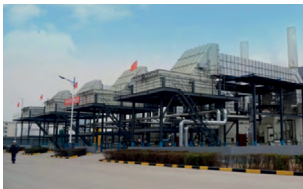
Figure 27: Titan 130 conventional combustion gas turbine packages operating with COG
